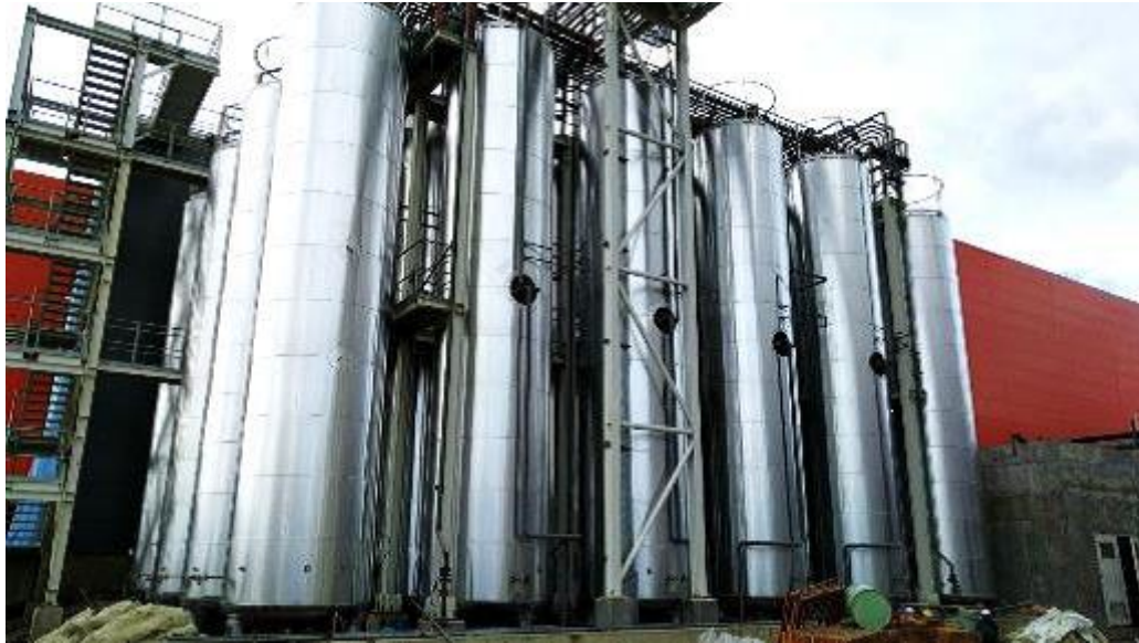
Tanks at the Utility and Refinery building where palm oil is processed
